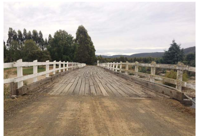
Figure 33: Amortised Wooden Bridge Needing to be Replaced
