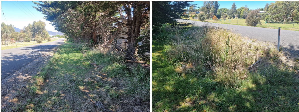
Figure 5: Western and eastern views along existing stormwater disposal in Frank Street including headwall
