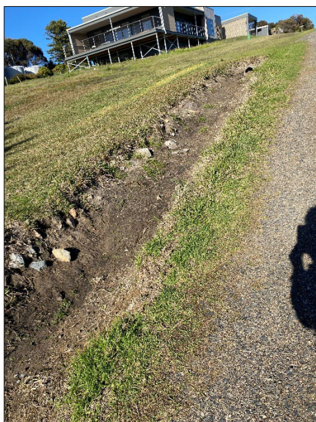
Photo 4 Legge St Stormwater Infrastructure (BODC)
